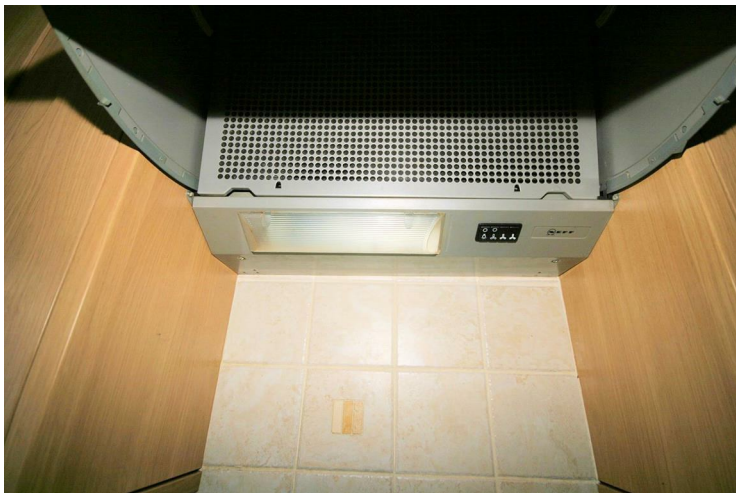
View of Extractor Fan
