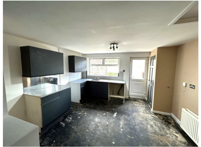
Separate kitchen area extension fitted with base and wall units. Inset sink. Door to outside.
